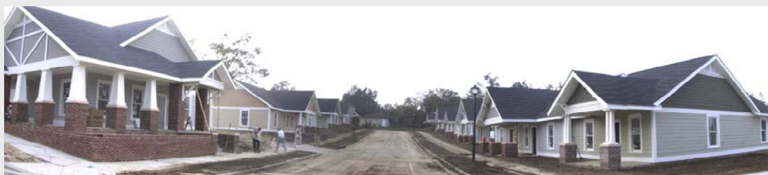
New construction of housing commenced on the property once occupied by Morningside public housing units. New construction on the adjacent units will begin in the next fiscal year.
