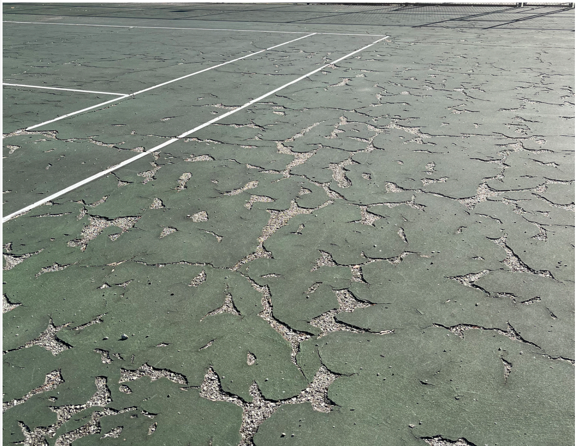
Tennis Court Condition at Hester Park
