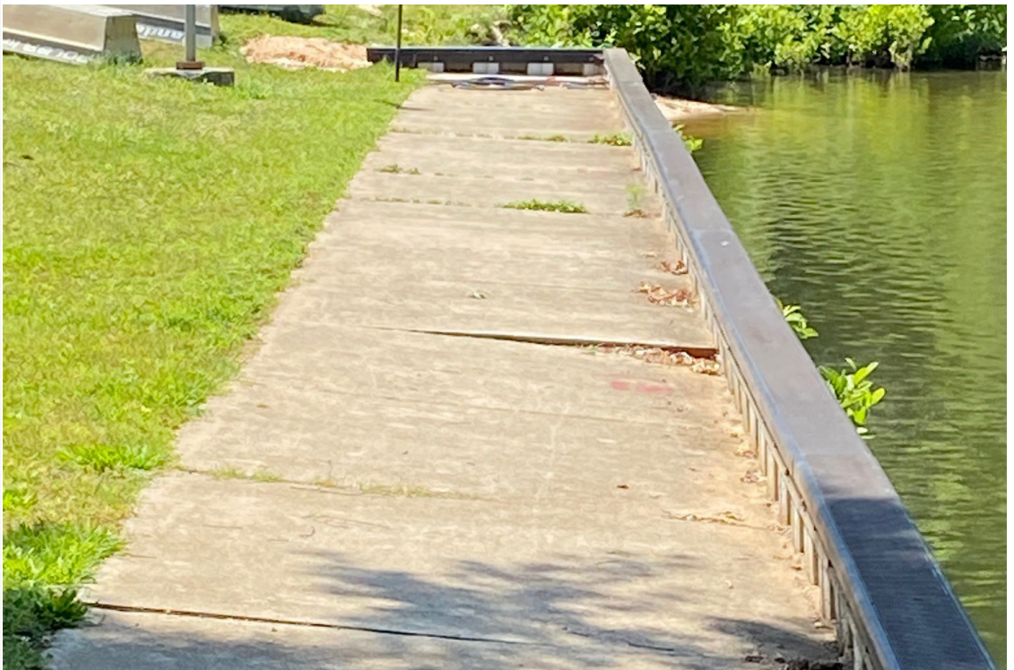
Failing Bulkhead at Lake Townsend Marina
