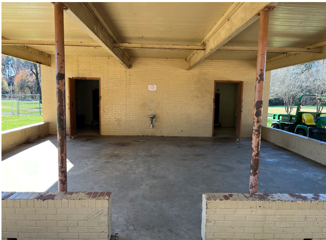
Restroom Conditions at Lindley Park
