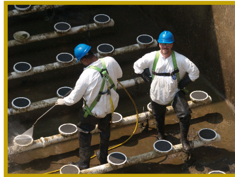
Routine facility maintenance by wastewater staff
