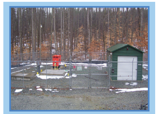
Reserve Lift Station
