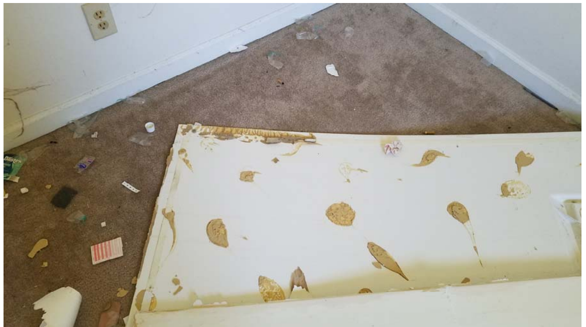
Example of wall glue and drywall/patch throughout each unit.
