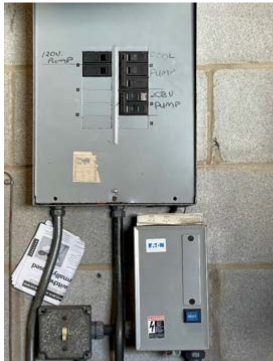
Figure E21 – Pump Room Panel
