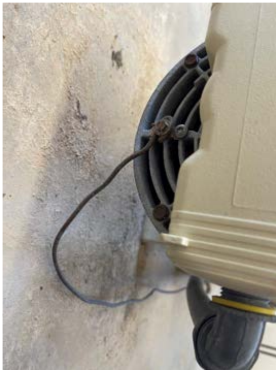
Figure E3 – Bonding Conductor and Lug
