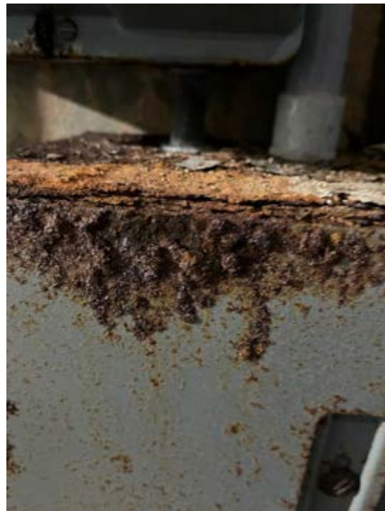
Figure E13 - Panel Degradation
