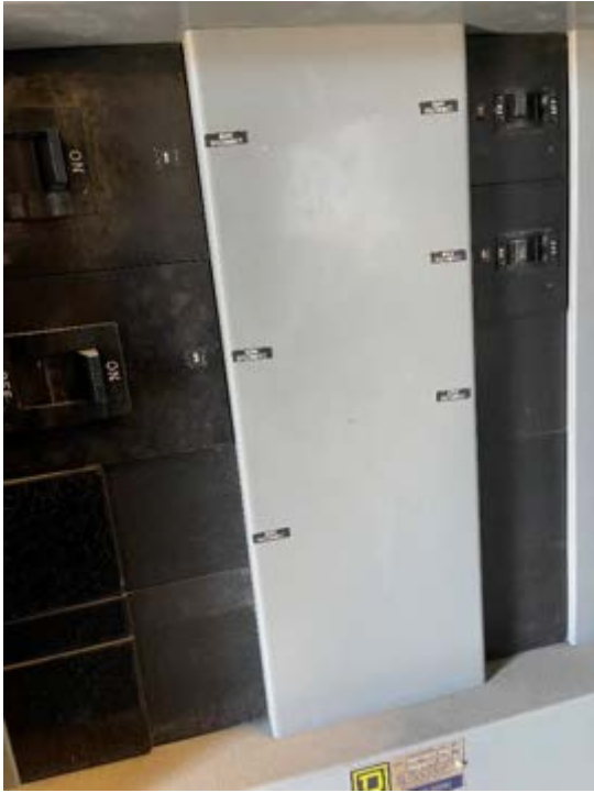
Figure E7 – Smith Center Main Electric Panel
