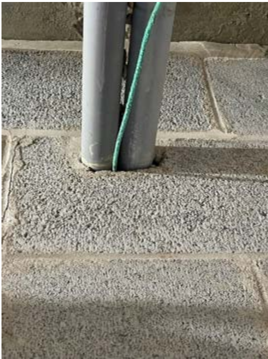
Figure E14 - Bonding Wire to Electric Room
