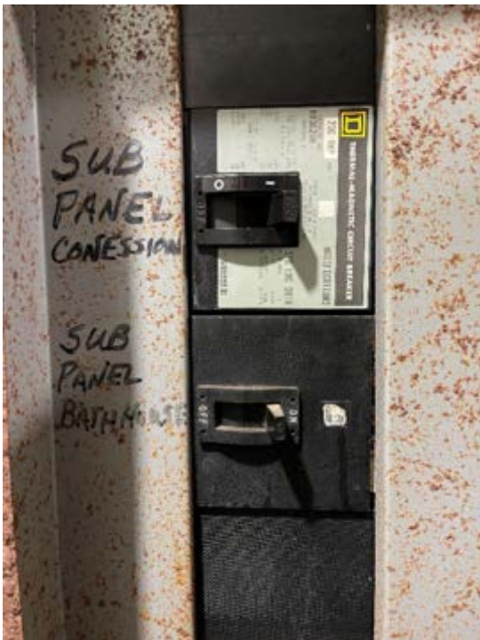
Figure E12 - Surface Rusting
