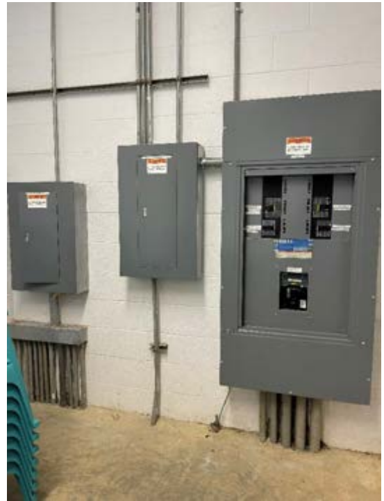
Figure E2 – Main and Branch Panels
