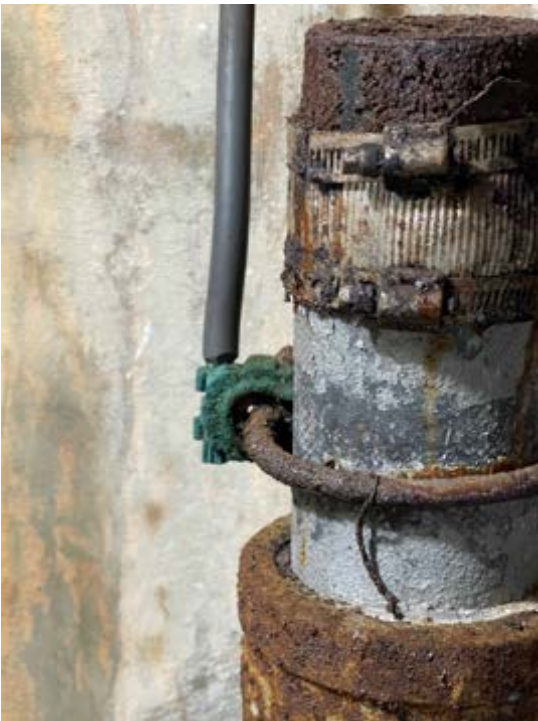
Figure E16 - Bonding Means Incorrect and Corroded
