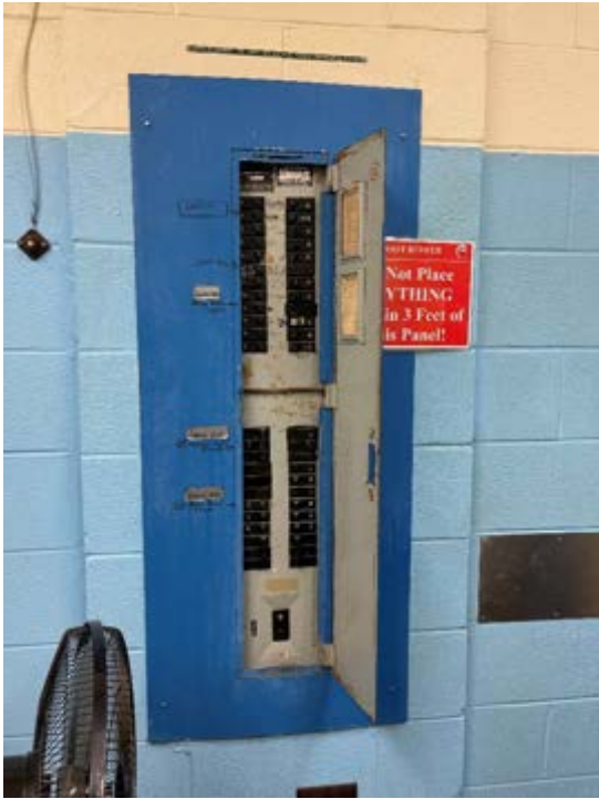
Figure E20 – Warnersville Main Electric Panel
