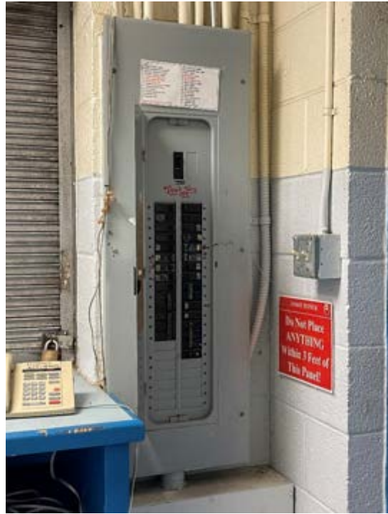
Figure E19 – Branch Panel in Pool House
