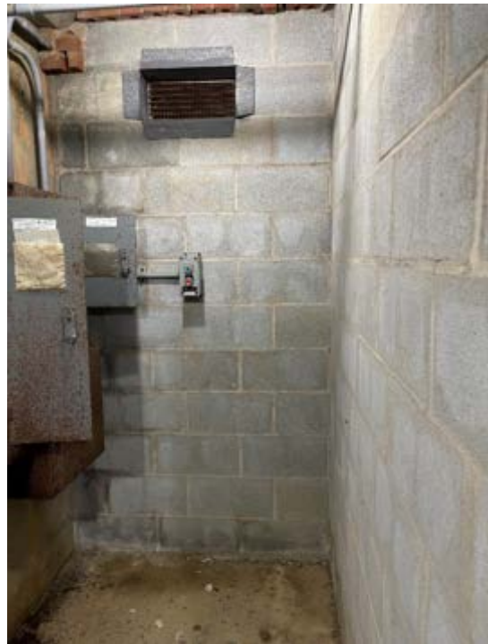
Figure E17 – Air Supply Louver from Pump Room
