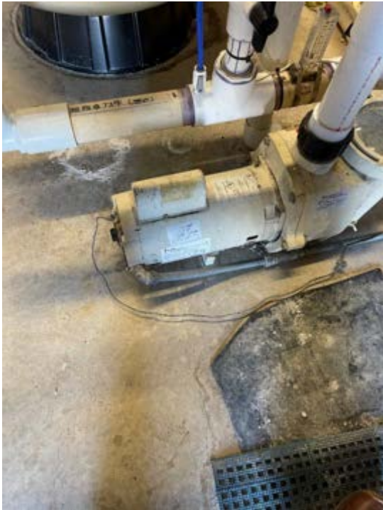
Figure E9 – Bonding Conductor at Pump
