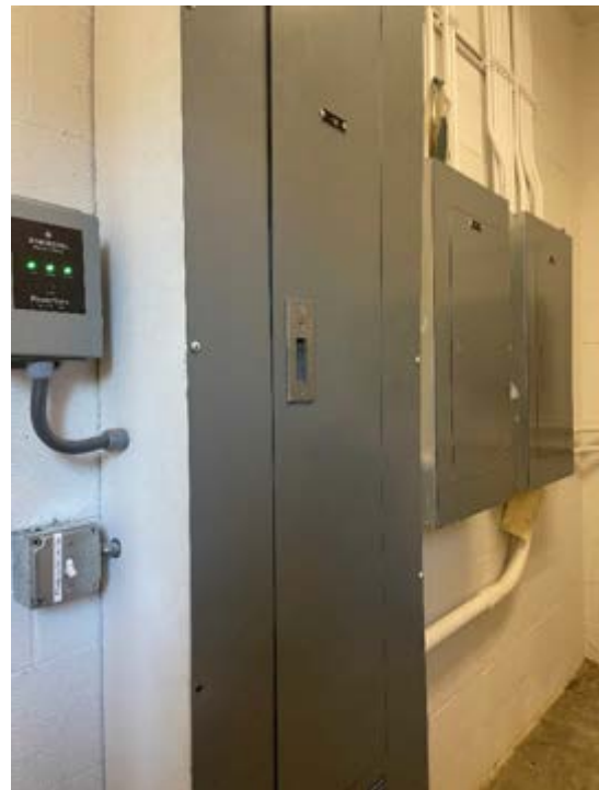
Figure E5 – Main and Branch Panels
