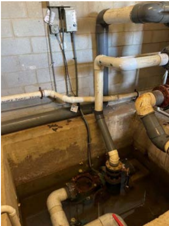
Figure E22 – Pit in Front of Panel and Controls
