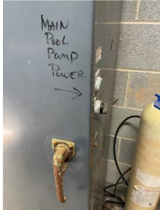
Figure E24 – Cabinet Corrosion
