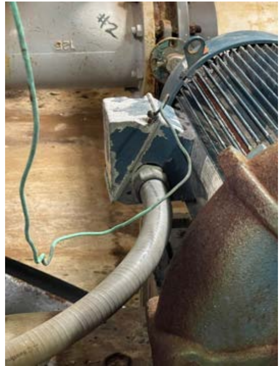
Figure E15 – Corrosion at Pool Pump Bonding Lug
