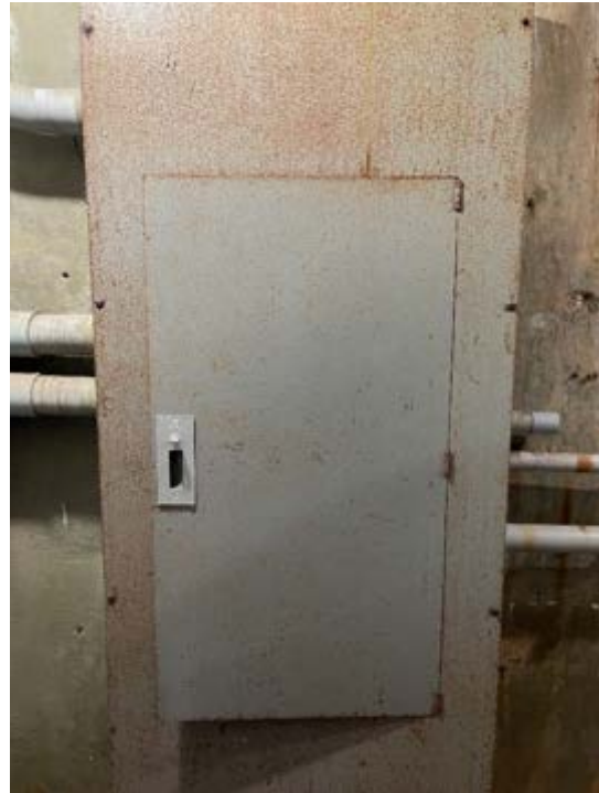
Figure E11 - Main Electrical Panel
