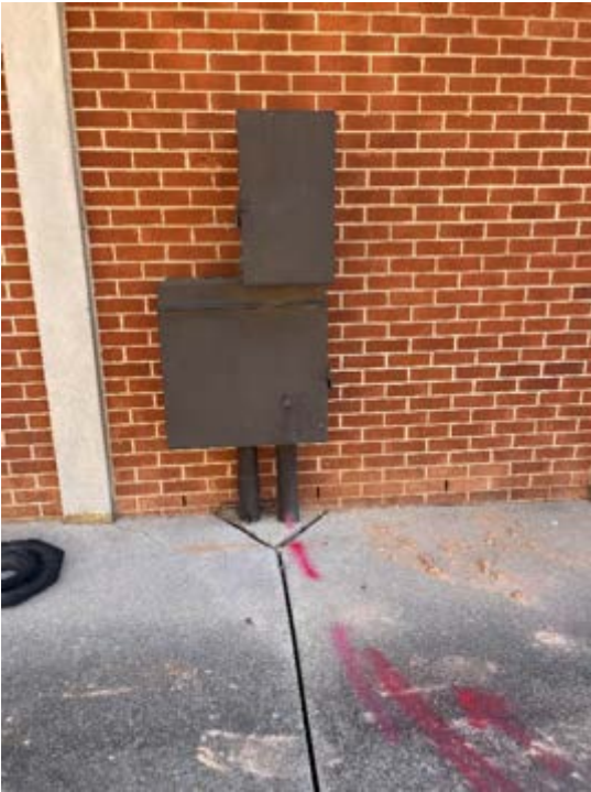
Figure E23 – Peeler Electric Service
