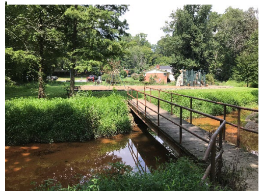
Figure 9 Aging infrastructure at Twin Lakes Park
