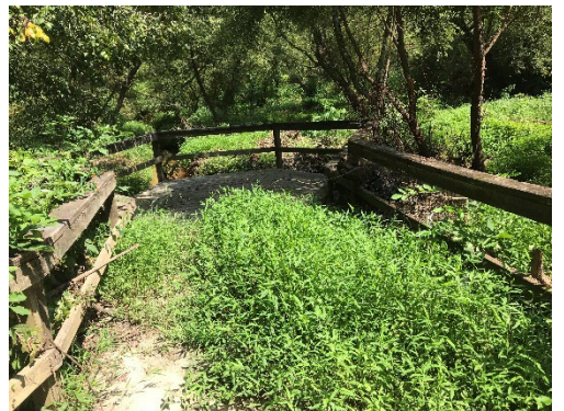
Figure 8 Deteriorated boardwalk at Pinecroft Lake Park
