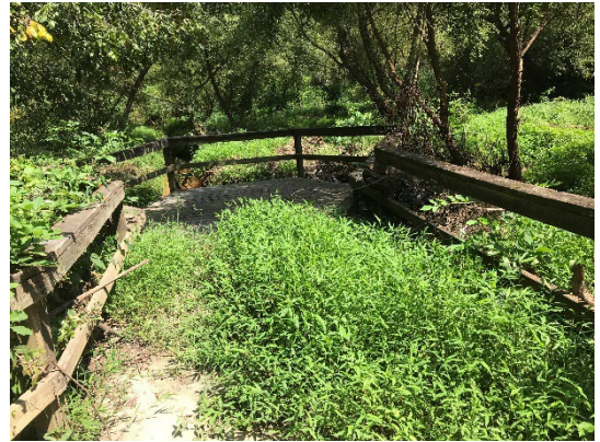
Figure 4 Overgrown vegetation on deteriorated overlook platform at Pinecroft Lake Park
