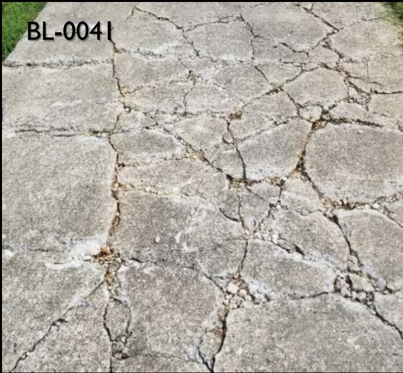
Lake Daniel greenway surface damage
