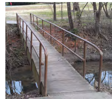
Undersized greenway bridges do not meet current standards and are barely wide enough for two pedestrians to pass each other comfortably.
