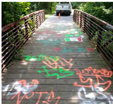
Graffiti is removed as soon as possible from the greenways, especially when it is done in a profligate manner, such as on this greenway bridge.
