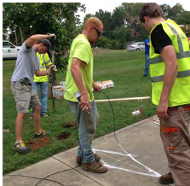
Permanent counters being installed on the Lake Daniel Greenway as part of the NCDOT Pilot Bicycle and Pedestrian Counting Program.
