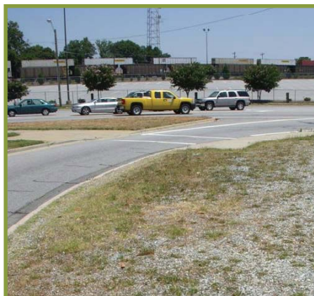
Lack of Sidewalk Connections
