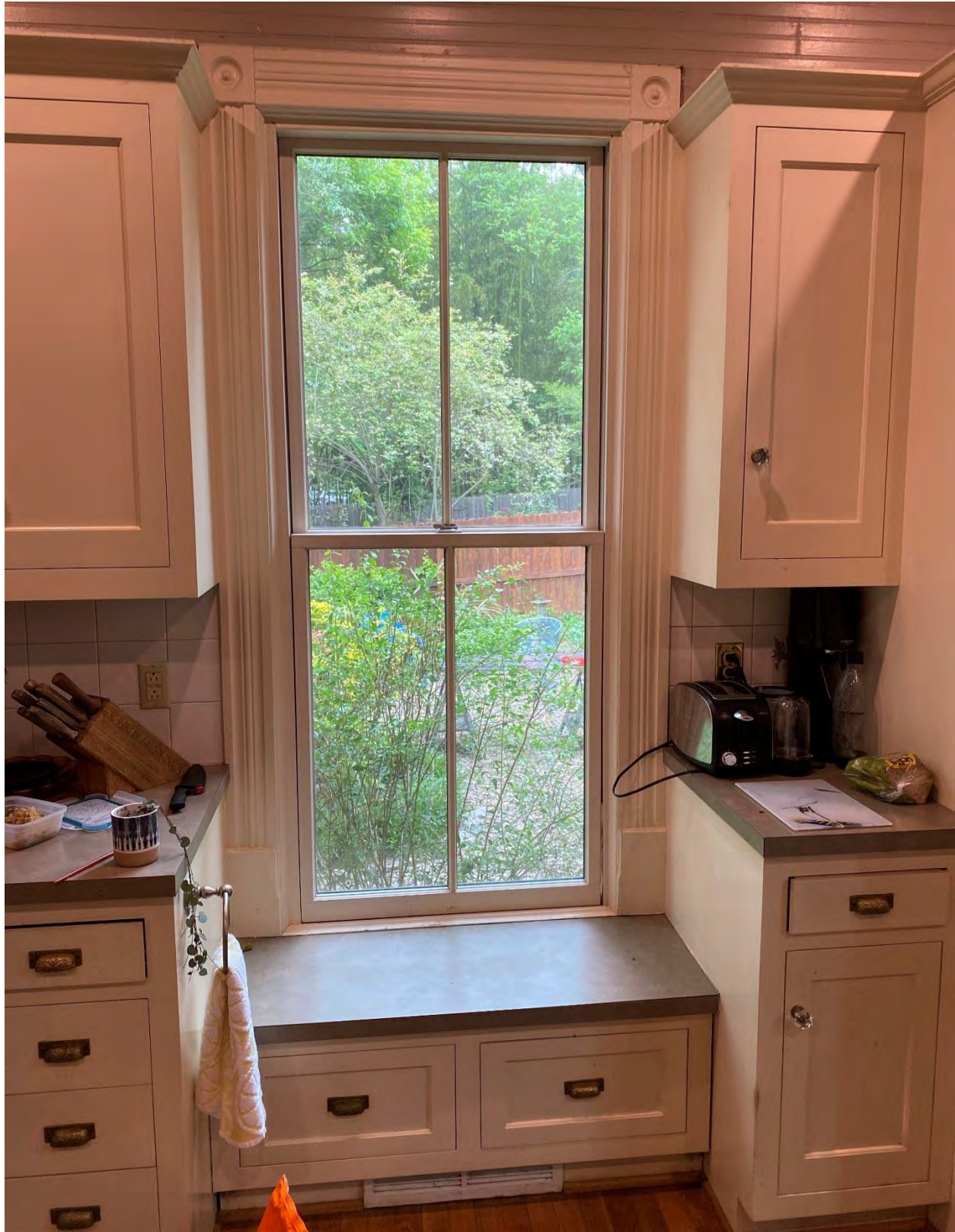
Figure 6 – 924 Carr St. rear elevation 1990's replacement window – external wood grids
