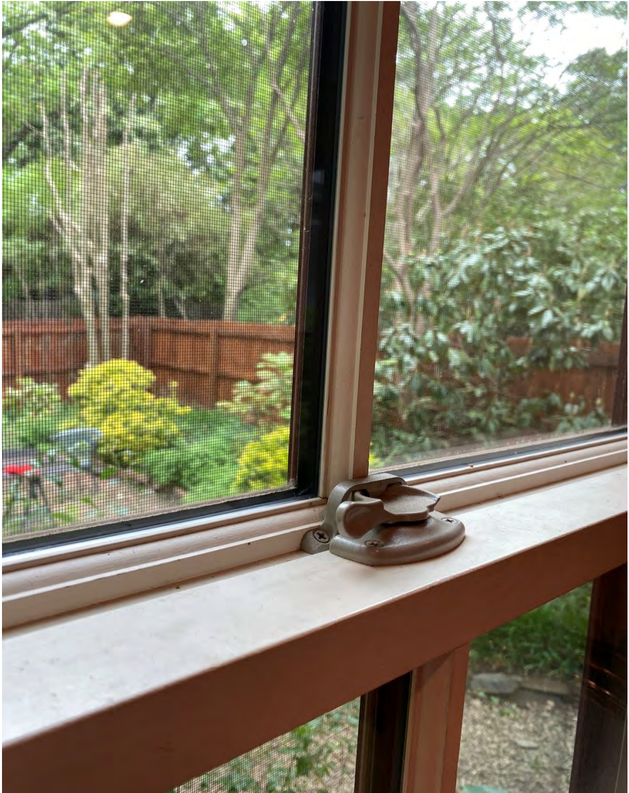
Figure 7 – 924 Carr St. rear elevation 1990's replacement window – external wood grids
