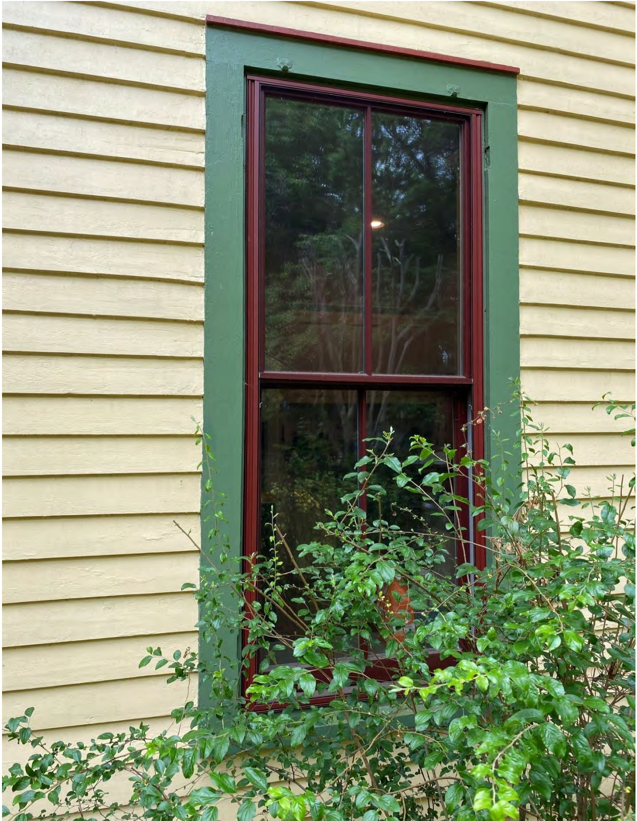
Figure 8 – 924 Carr St. rear elevation 1990's replacement window – external wood grids
