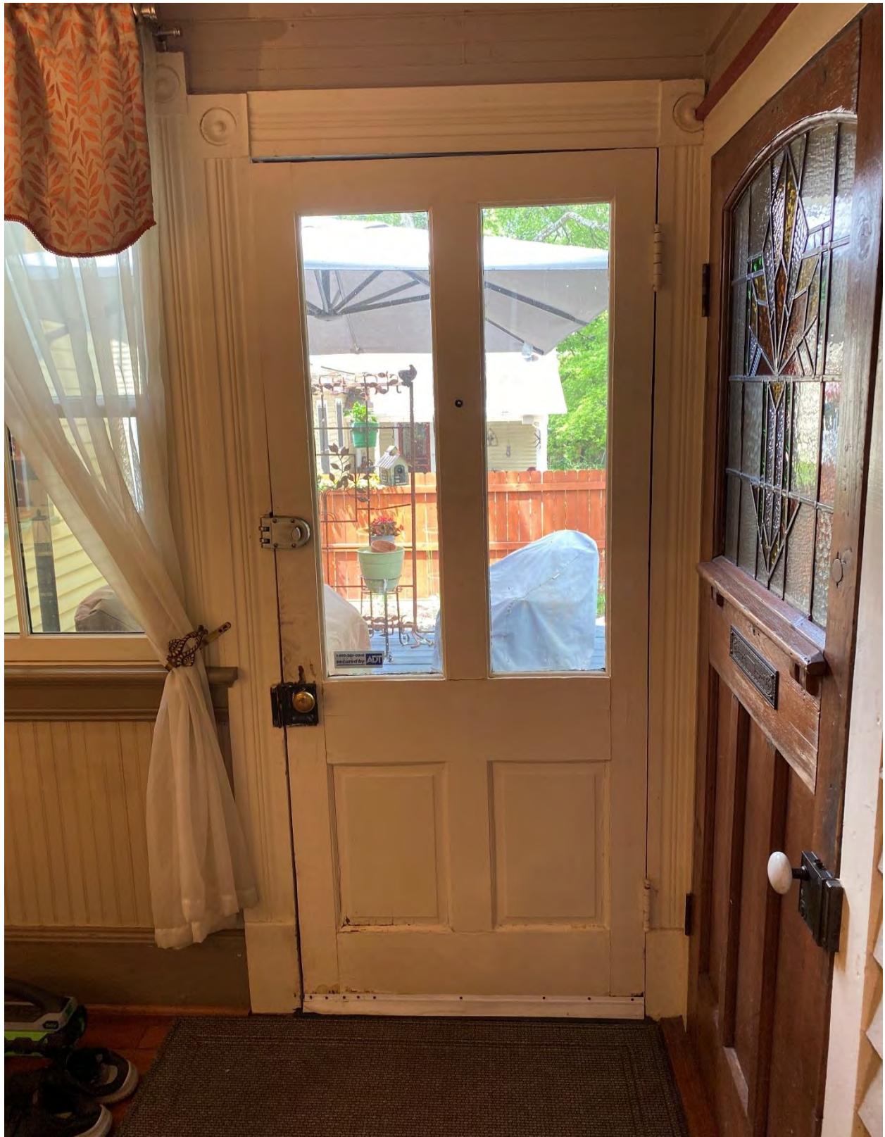
Figure 25 – 924 Carr St. rear side entrance inappropriate modified door
