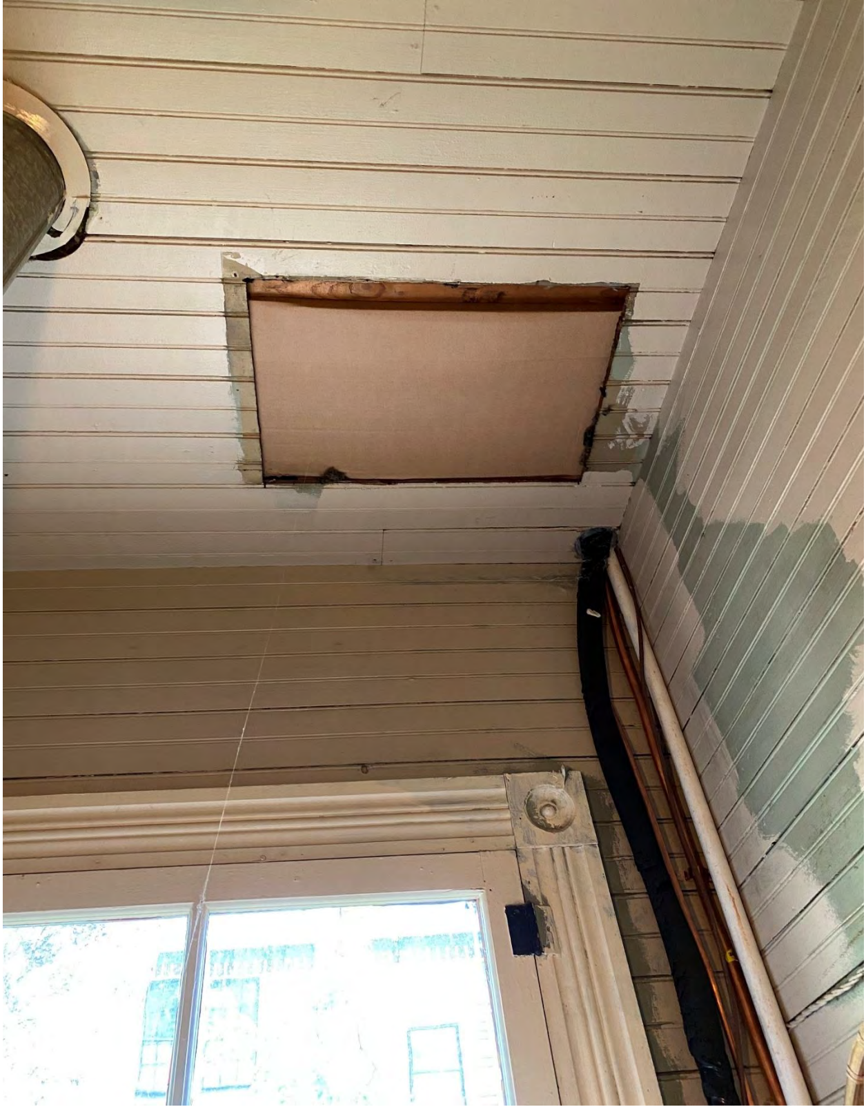
Figure 16 – 924 Carr St. storage room ceiling patch
