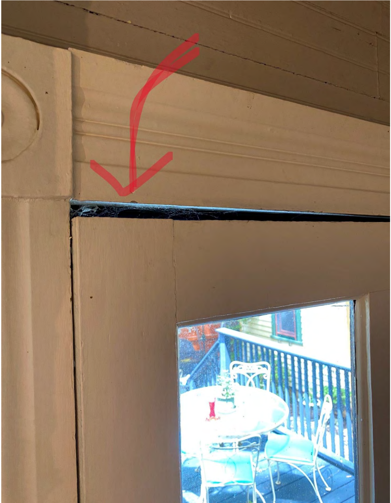
Figure 26 – 924 Carr St. rear side entrance door leakage
