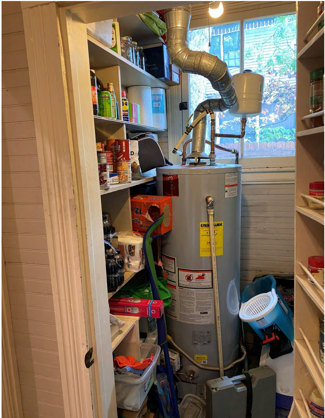
Figure 17 – 924 Carr St. storage room obstructed by water heater
