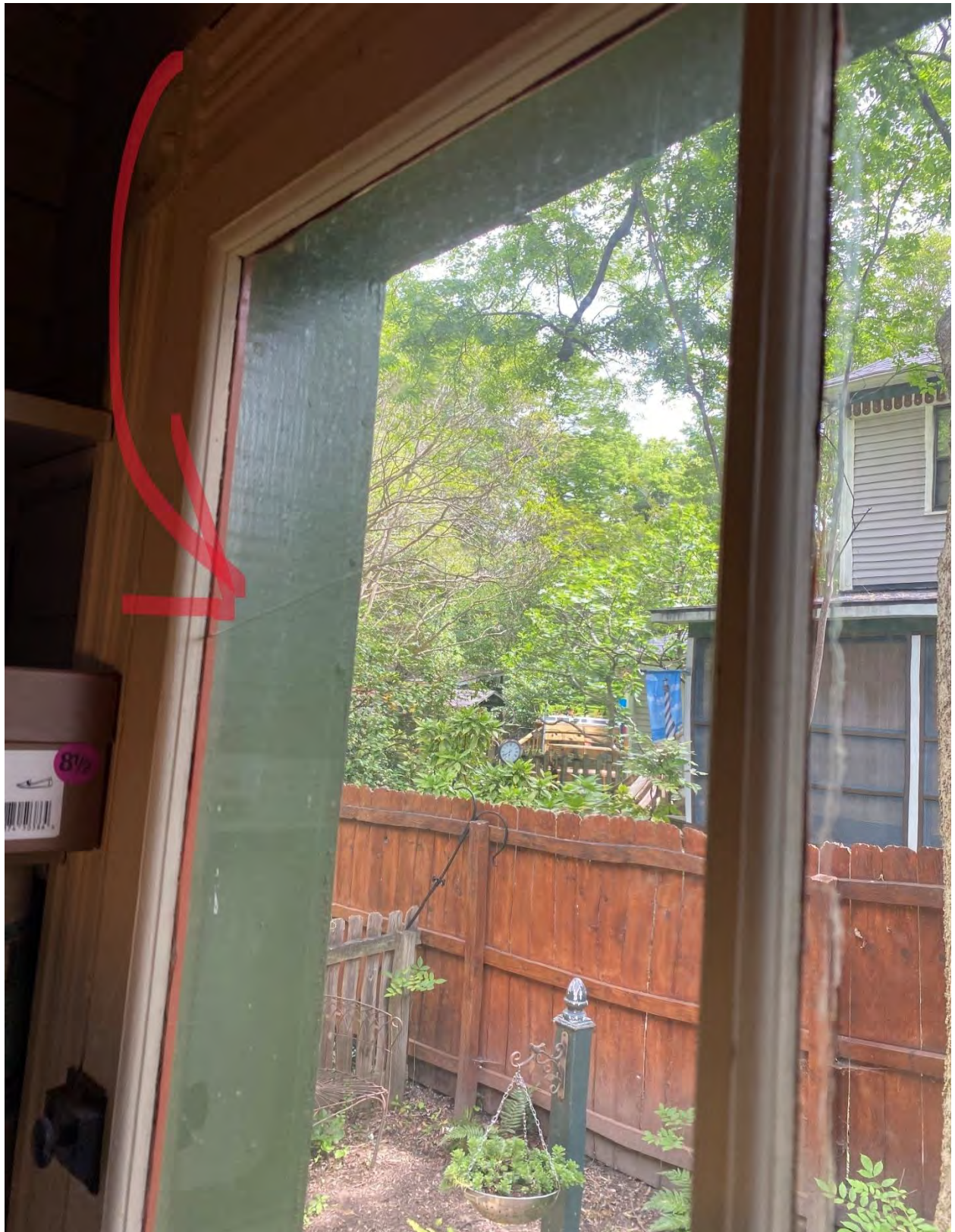
Figure 19 – 924 Carr St. broken window in unheated storage room
