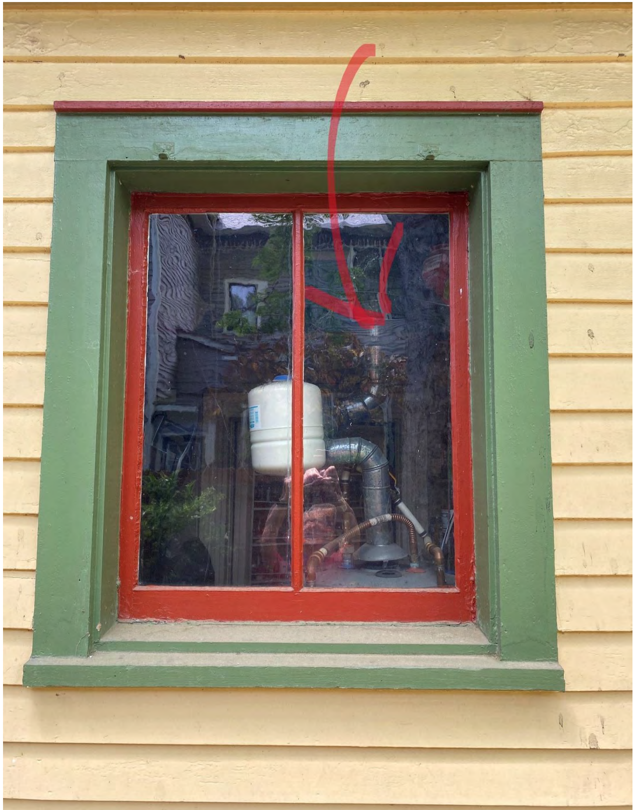
Figure 20 – 924 Carr St. broken window in unheated storage room
