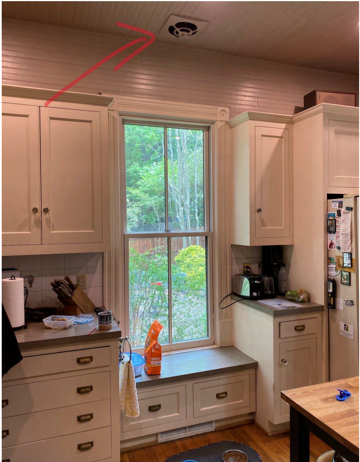
Figure 9 – 924 Carr St. vestigial cookstove exhaust fan
