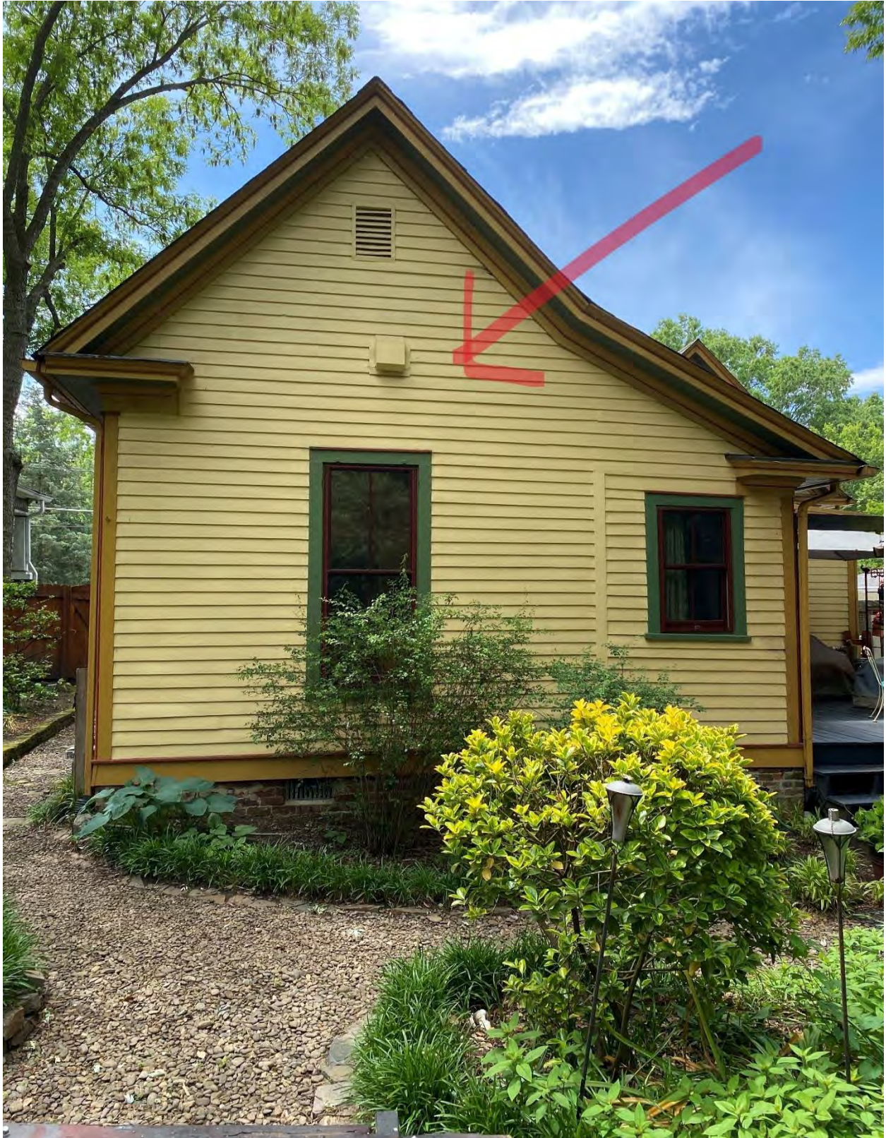
Figure 10 – 924 Carr St. vestigial cookstove exhaust fan
