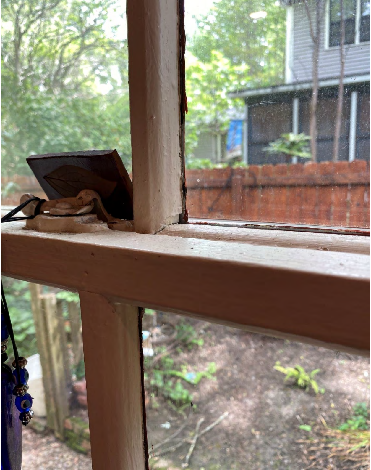
Figure 12 – 924 Carr St. side elevation reworked window, possibly not original location
