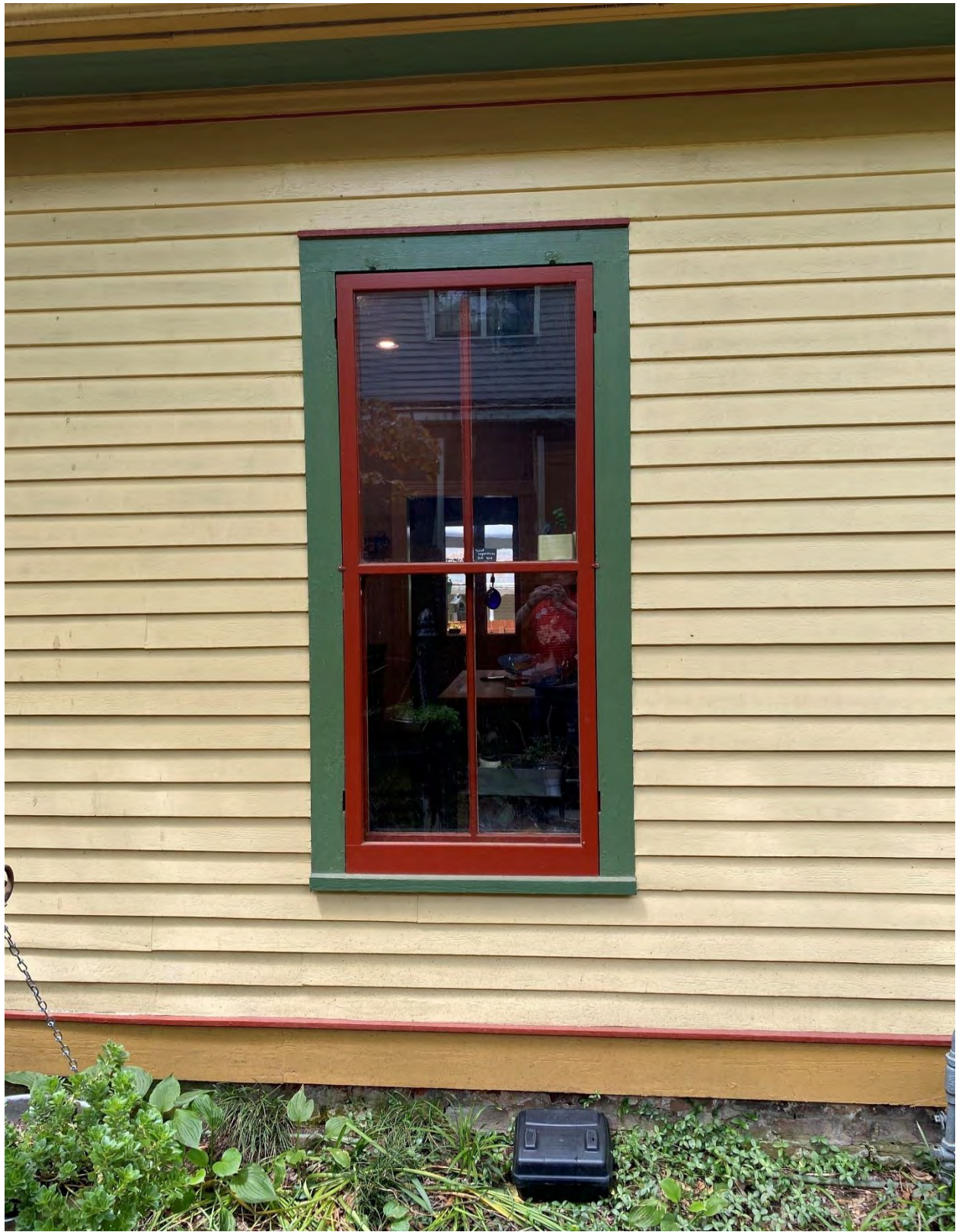
Figure 13 – 924 Carr St. side elevation reworked window, possibly not original location
